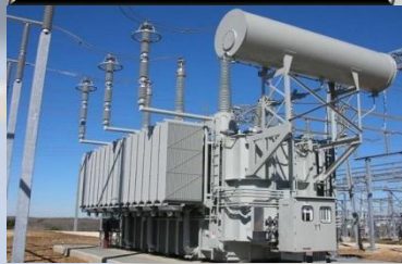
Substation Up to 132Kv
